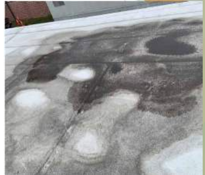
Roof system surface deterioration
