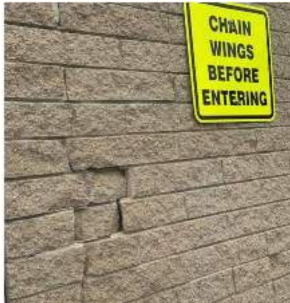
Masonry cracks / damage
