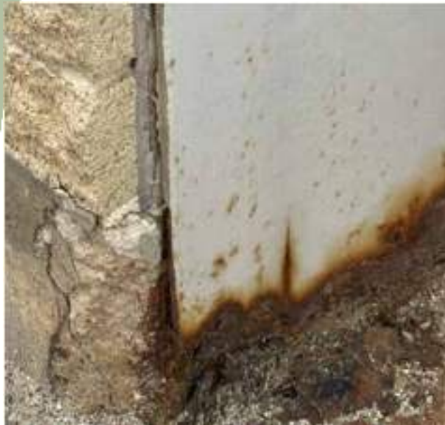
Corrosion impacting structural integrity
